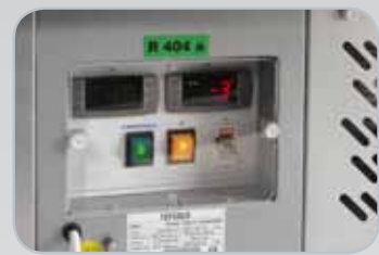
2 thermostats for switching from cooler to freezer
